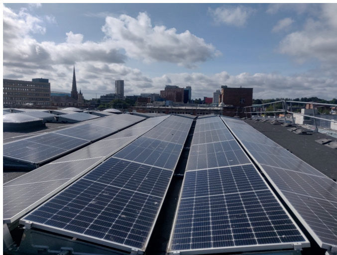
Figure 14 – Solar panels on the roof of Central Library
